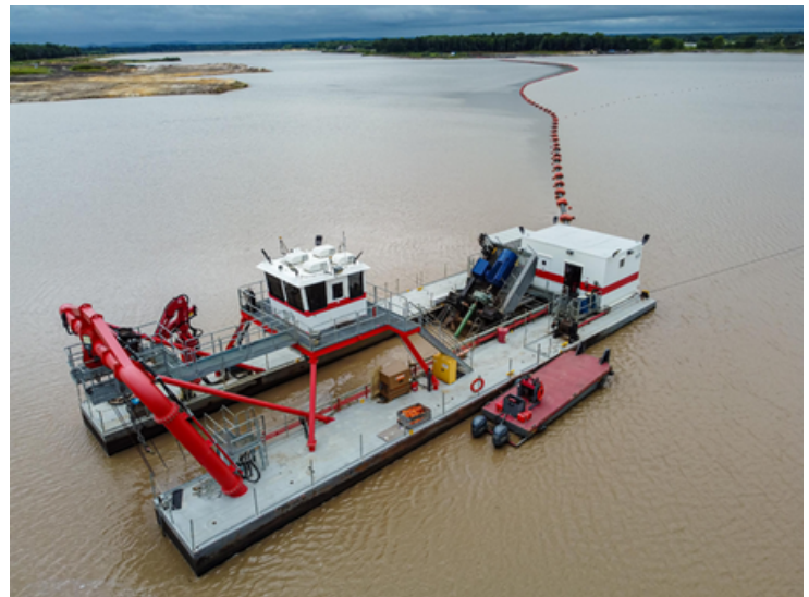
Dredging equipment removes sand from riverbeds and lakes. Rivers and lakes often concentrate durable quartz grains that meet the strict requirements of industrial sand.
